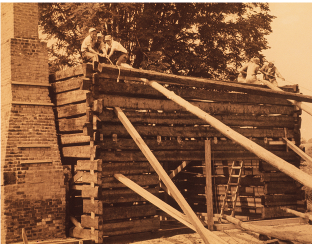
Workmen lift the shaped pine logs into place on the second story of the reconstructed Vance House. Ca. 1960
