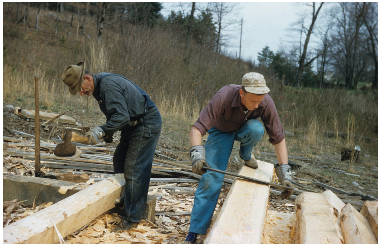
Workmen use traditional tools to shape the logs for the outer walls of the reconstructed Vance House. Ca. 1960.
